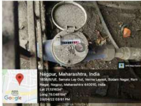
NMC Water Meter
