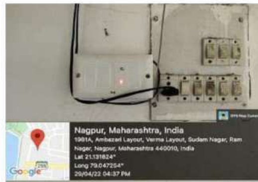
Sensor based lighting system installed in college
