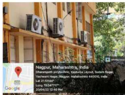
AC Condensers in shade
