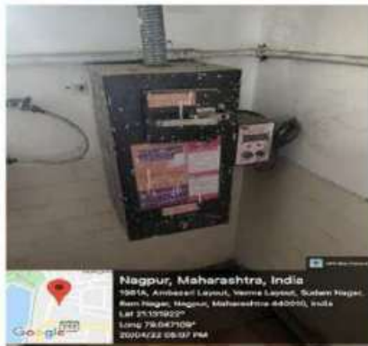
Incinerator machine in Girl's Common Room
