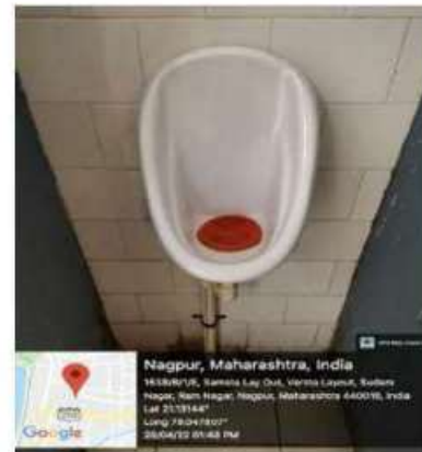
Flush less Urinals installed in college
