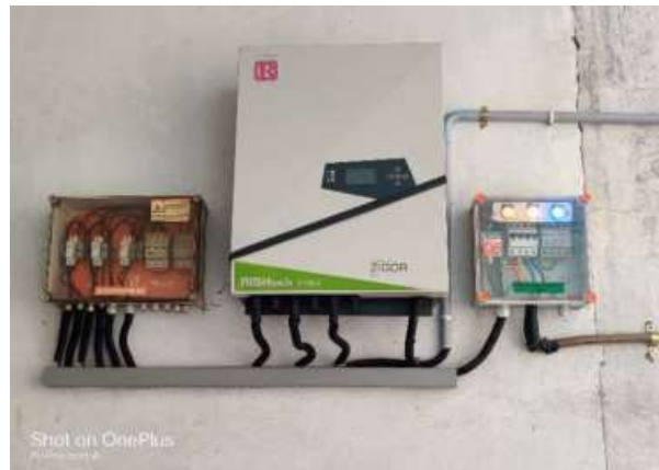
Figure 4: On Grid solar power converter installed in the building
