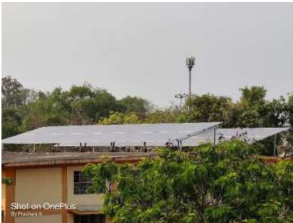
Figure 2: Solar panels installed on the Science Building
