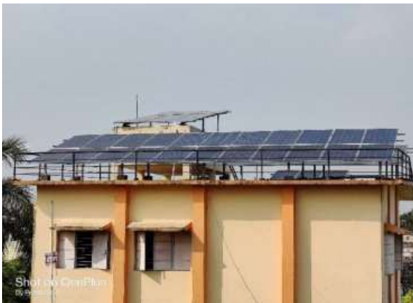
Figure 3: Solar panels installed on Home Science Building
