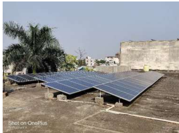
Figure 1: Solar panels installed on Administrative Building
