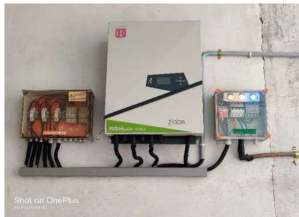
Figure 4: On Grid solar power converter installed in the building
