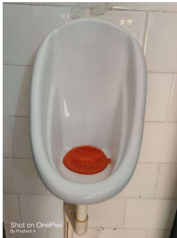
Figure 1 &2: Flush less Urinals installed in the Male Urinals of the College
