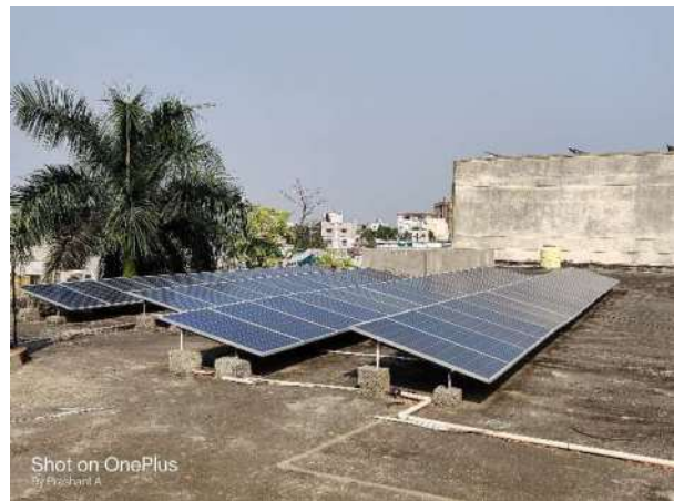
Figure 1: Solar panels installed on Administrative Building
