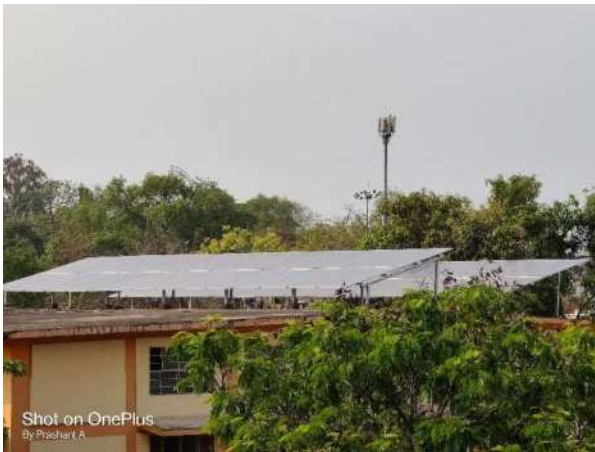
Figure 2: Solar panels installed on the Science Building
