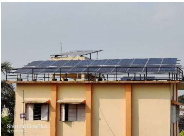
Figure 3: Solar panels installed on Home Science Building
