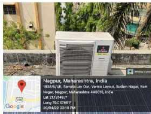
AC Condensers exposed to direct sunlight
