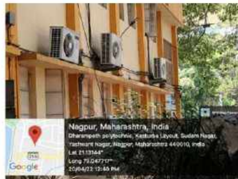
AC Condensers in shade
