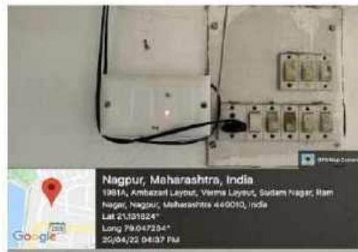
Sensor based lighting system installed in college
