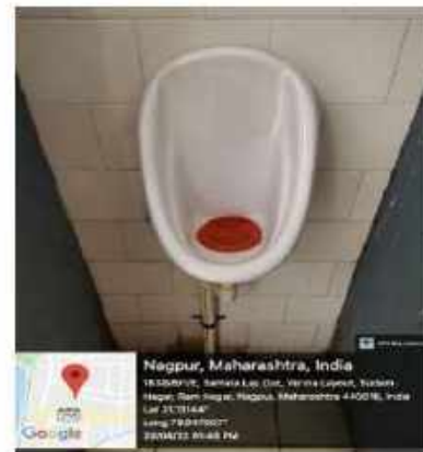
Flush less Urinals installed in college
