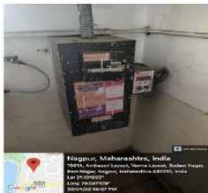
Incinerator machine in Girl's Common Room
