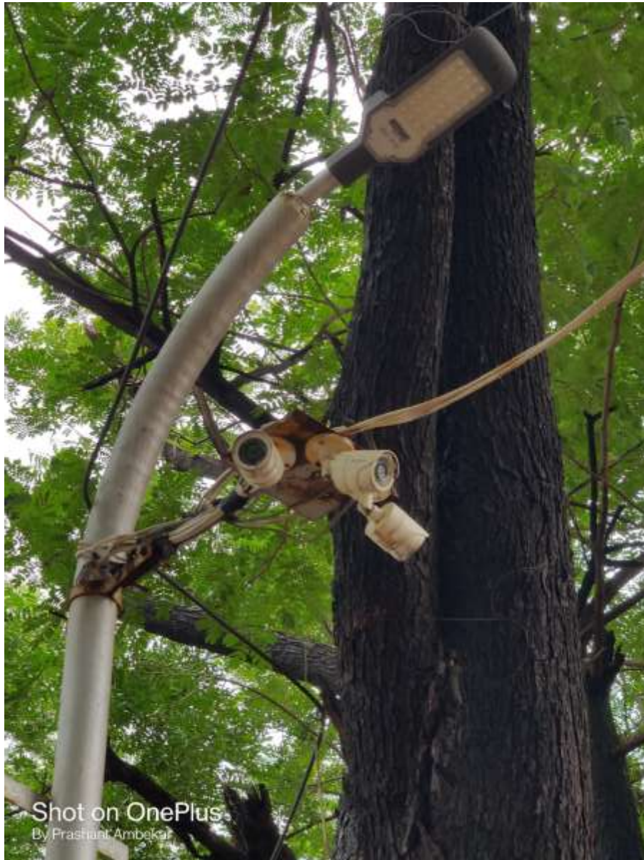
7.1.1. CCTV Cameras Installed
