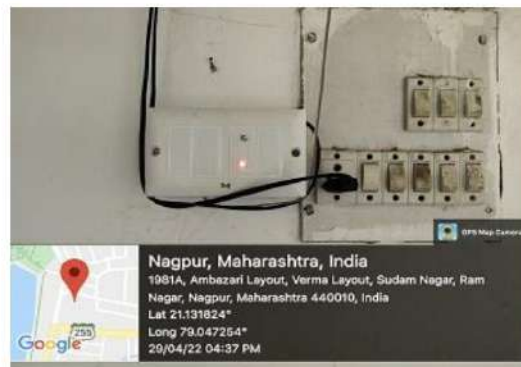
Sensor based lighting system installed in college
