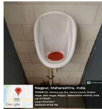
Flush less Urinals installed in college
