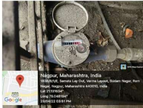
NMC Water Meter
