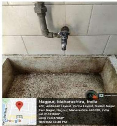
Taps to be replaced by Push Buttons / Faucets
