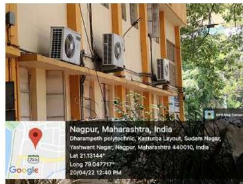
AC Condensers in shade
