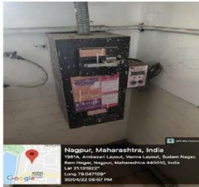
Incinerator machine in Girl's Common Room
